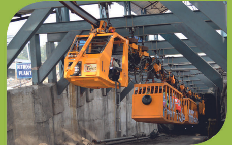
Installation of Monorail Man-riding system for transportation of workmen in Moonidih UG Mine: First time in India.
